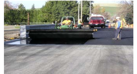
The geotextile fabric is placed prior to asphalt paving. The fabric will help prevent reflective cracking in the concrete.
