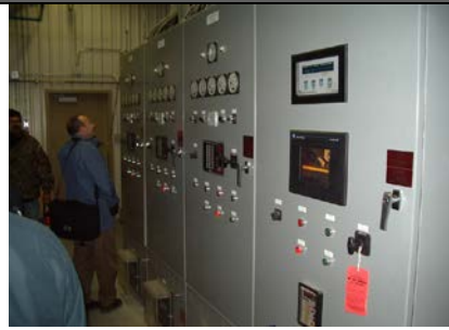
Inside a substation
