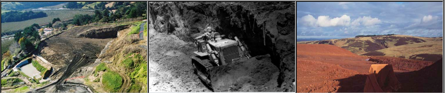
Borrow Pit – an area where material (usually soil, gravel or sand) has been dug for use at another location.
