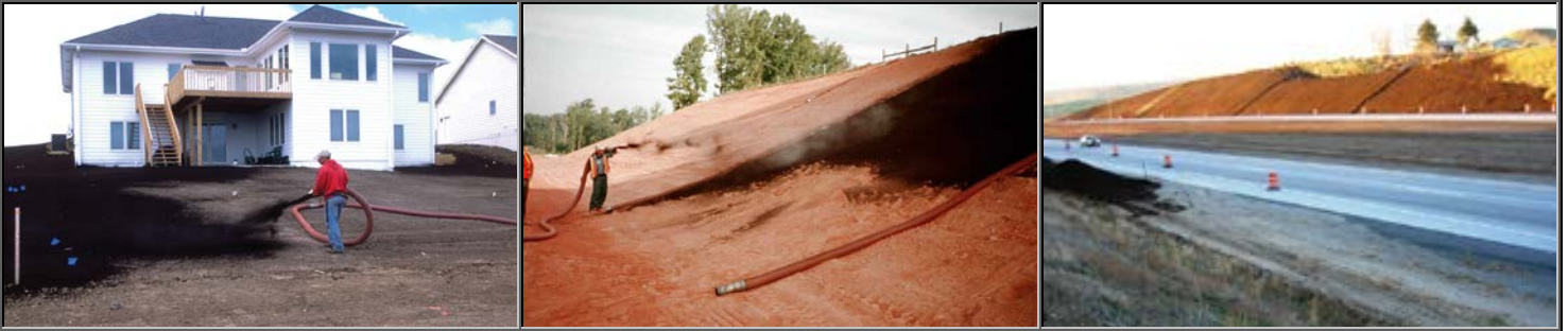
Compost Blanket – a 1 to 4 inch surface application of compost/mulch or a blend of both to protect areas with erosive potential.
