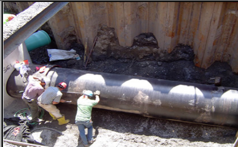
DIP, Ductile Iron Pipe – Water Main
