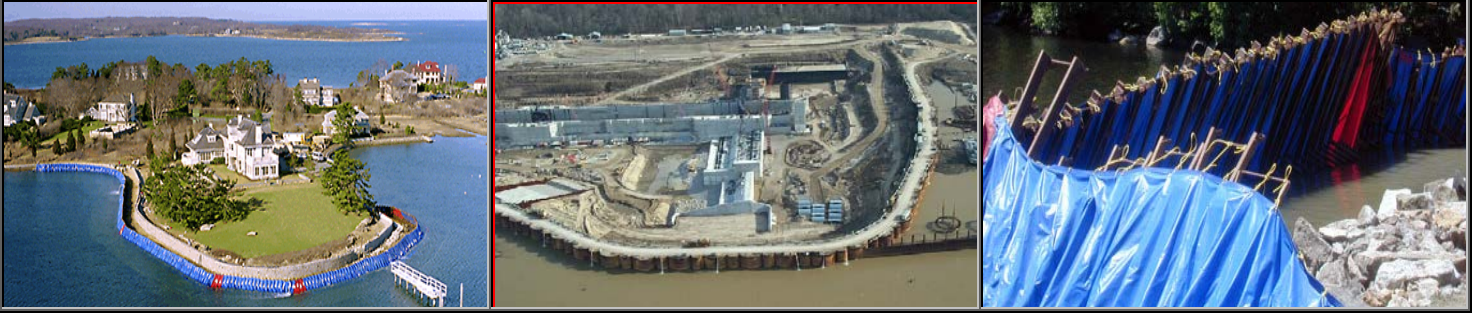
Cofferdam – a temporary barrier used to provide a dry work area below the water level.
