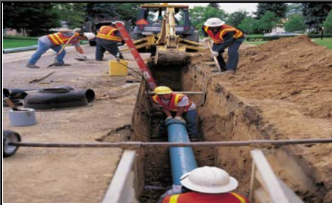
DIP, Ductile Iron Pipe – Water Main
